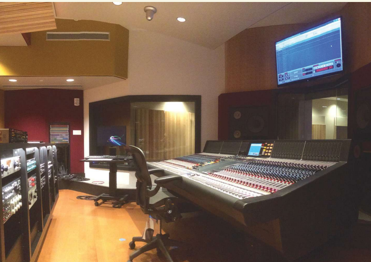
Studio 2 (formally named The Ark) is the second-largest facility in the new 10-studio complex. The control room houses a 48-channel Neve 88RS automated console and a tracking room with a Bosendorfer seven-foot grand piano and floor space for up to 30 live players.
