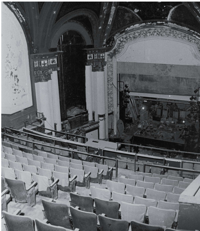
When Berklee purchased the theater from Bryant & Stratton Commercial School in 1972, the once-grand theater, with its gilded proscenium, vaulted ceiling, and box seats on the side walls, had fallen into disrepair.
